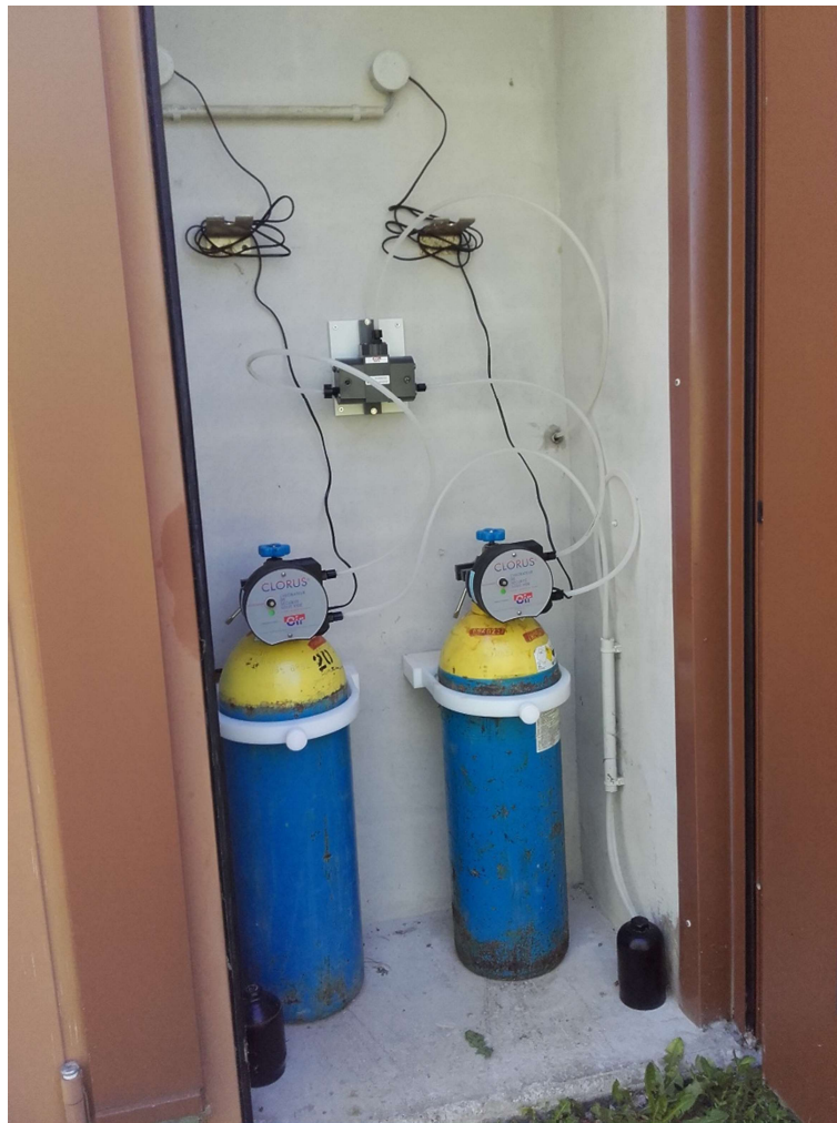
Figure 6 : Injection de chlore
